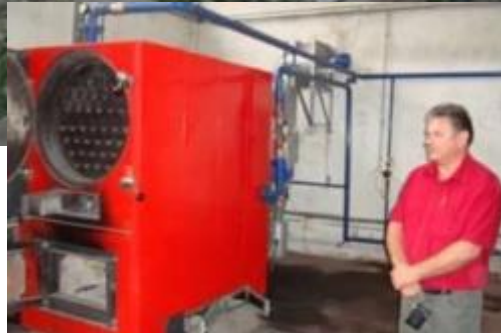
Biomass thermal plant Sfantu Gheorghe – Tega Company
